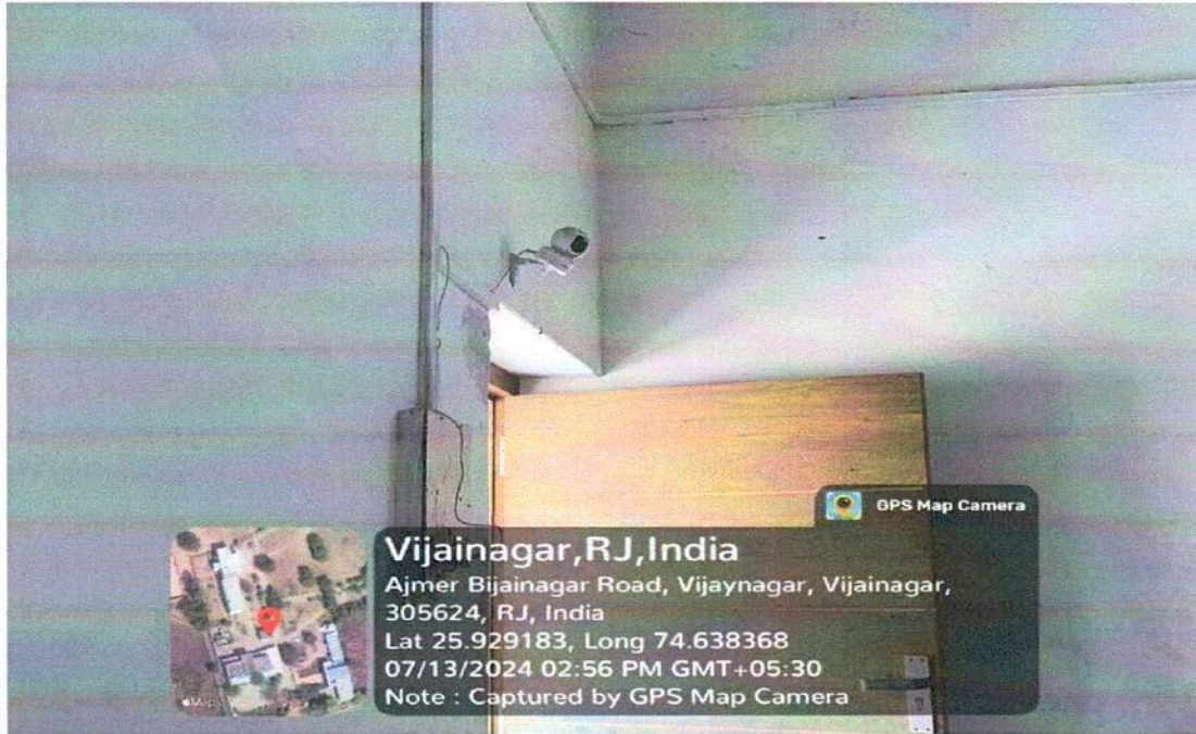
CCTV no 1 for security
