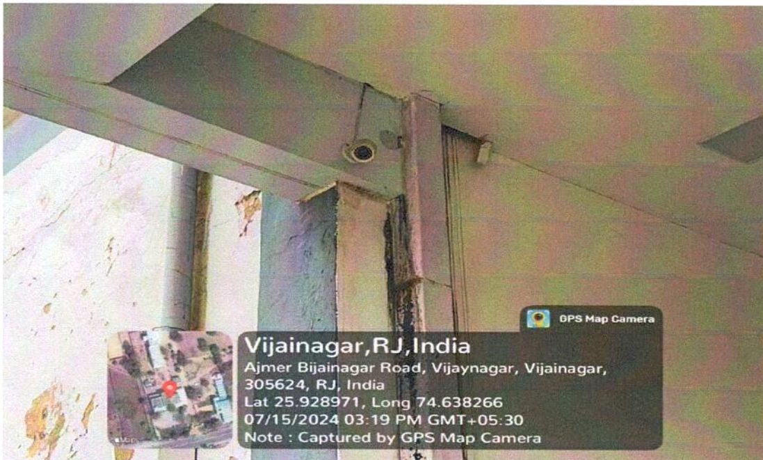
CCTV no 4 for security
