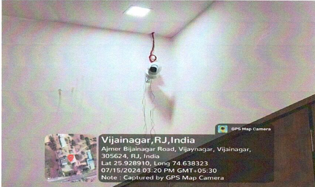
CCTV no 3 for security
