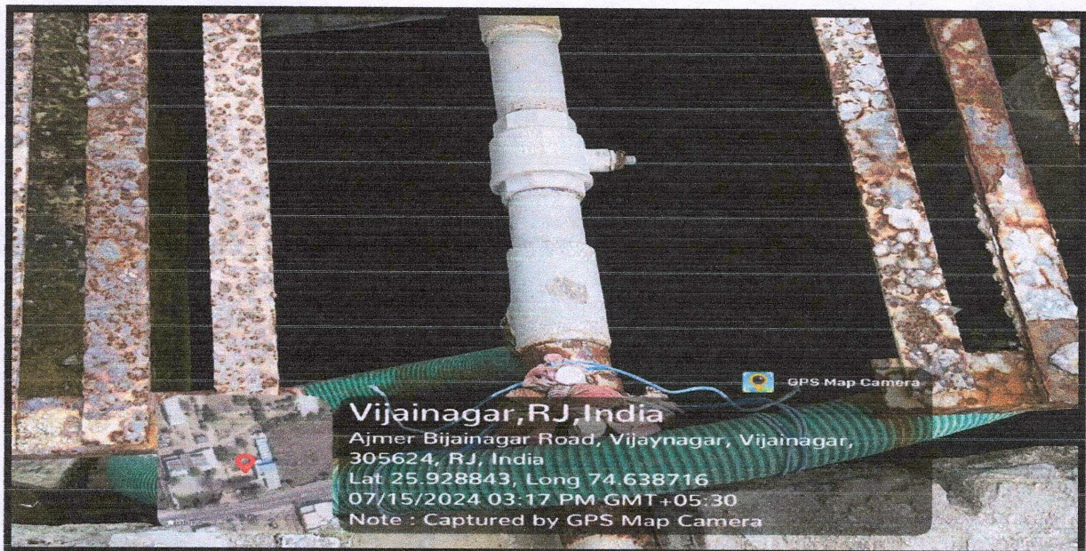
Water Harvesting Plant
